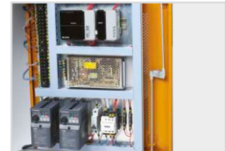
PLC (Programmable logic controller) and High Quality Electrical Components
